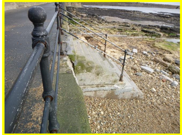
Steps in fair condition (/C0401C05)
