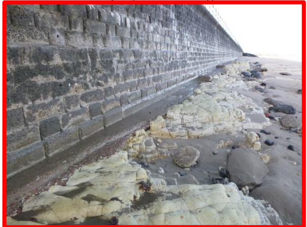
Evidence of abrasion to wall (/C0303C01)
