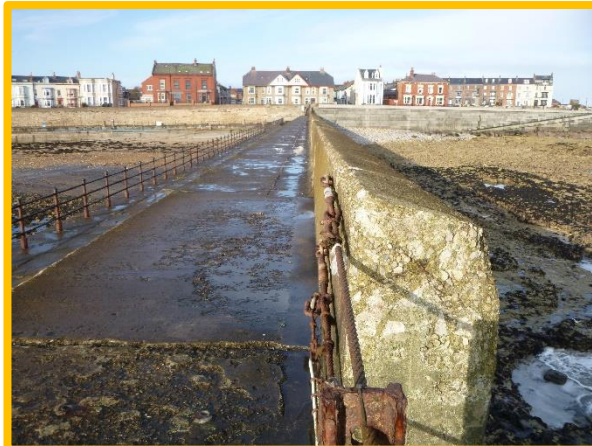
Spalling of concrete (/C0401C01)
