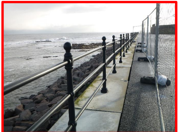
Evidence of movement of coping stones (/C0303C02)
