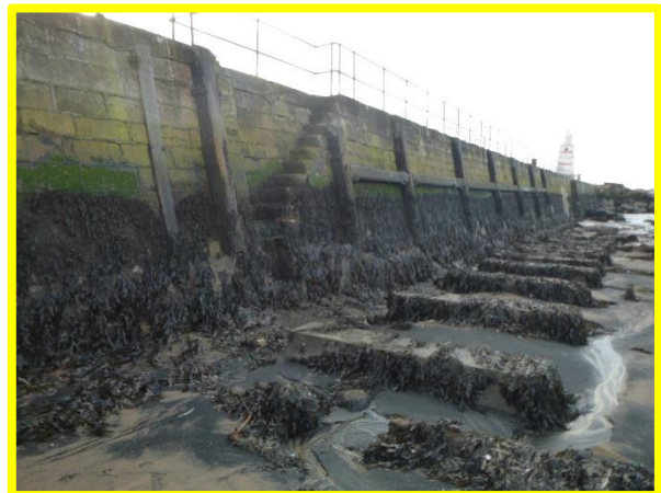
Inner face of North Pier – uneven profile suggesting potential settlement of masonry blocks (/C0401C06)
