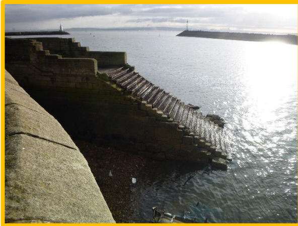
Damage to steps at former passenger ferry landing (/C0401C35)
