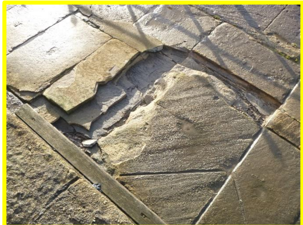
Cracking to the deck slab (/C0401C01)
