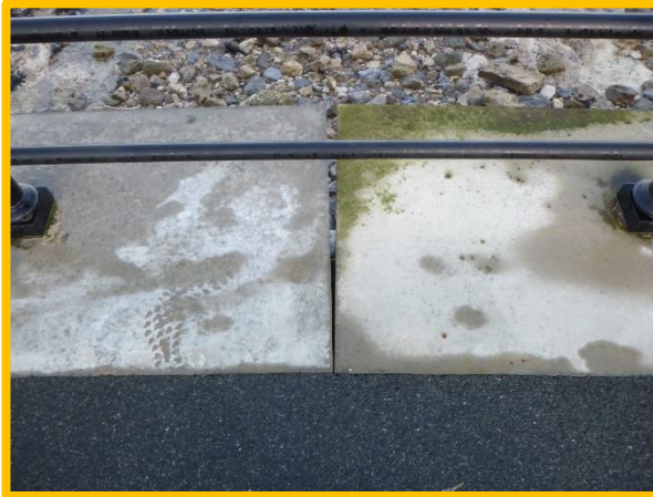
Missing flexible joint sealant (/C0303C02)
