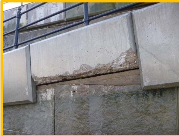
Damage to coping stones (/C0303C02)
