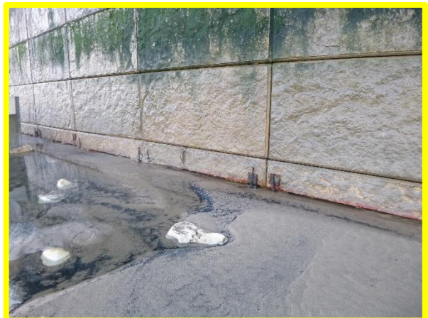
Exposed toe of wall (/C0303C01)
