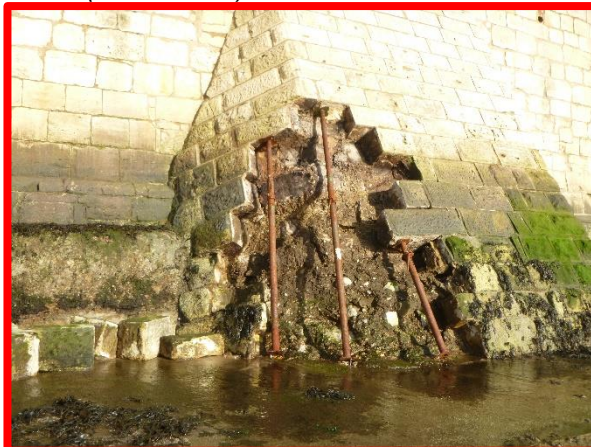
Significant defect to masonry abutment (/C0401C35)
