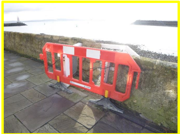
Beach access steps closed off (/C0401C35)
