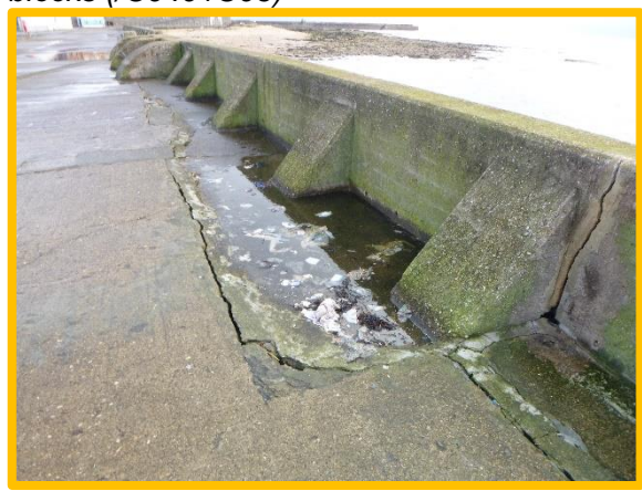
Cracking in parapet wall and deck (/C0401C34)
