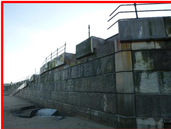
Missing coping stones (/C0303C01)
