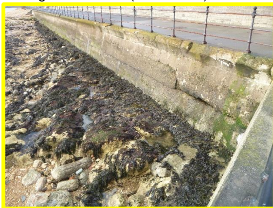
Damaged cope around handrailing fixing (/C0401C04)
