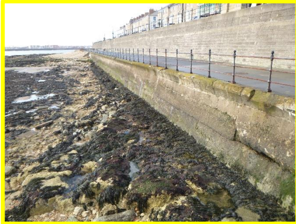
Damaged recurve cope (/C0401C05)
