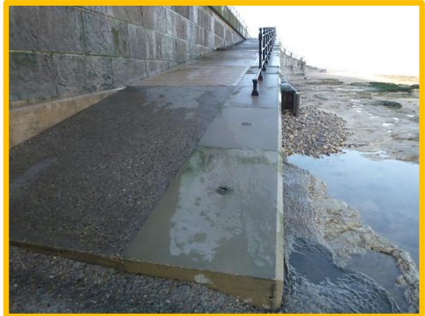
Missing section of handrail (/C0303C04)
