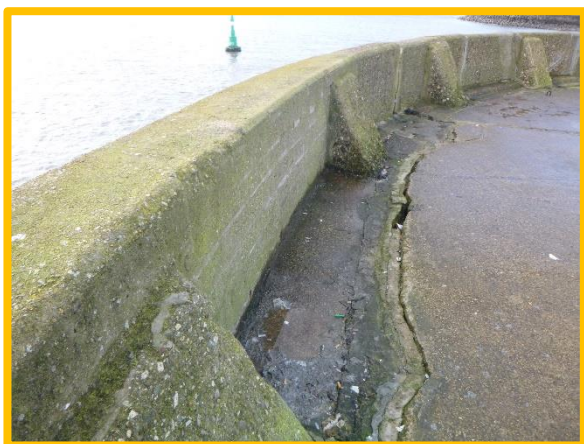
Cracking in parapet wall and deck (/C0401C34)
