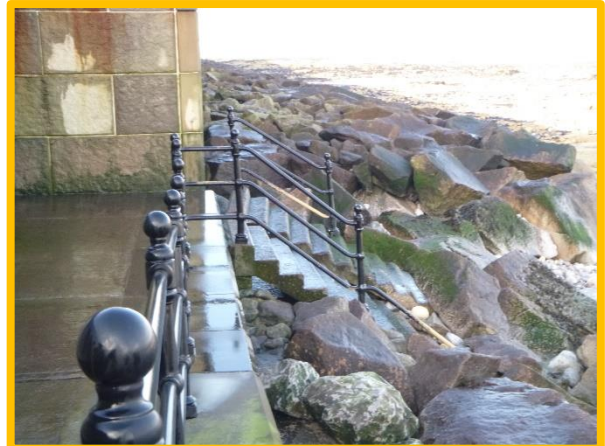
Extensive evidence of rock movement notably around failed access steps. (/C0303C04)
